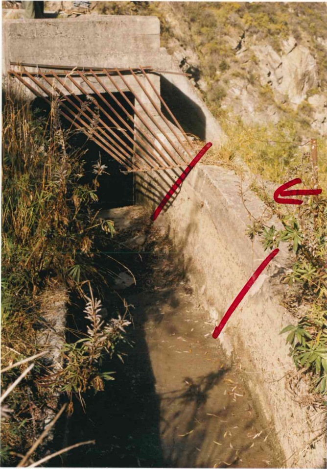
View of the race inlet to the desilting structure. The area marked has moved and as a result of the downstream erosion there is now little lateral support.
