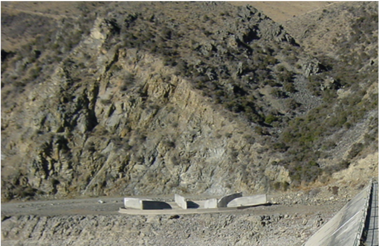
Figure 6 View of quarry face above left abutment bell mouth bench showing shear zones
