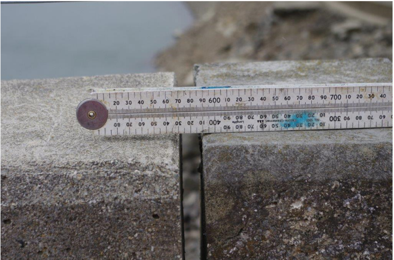
Figure 17 Offset at TL perimetric joint c2015
