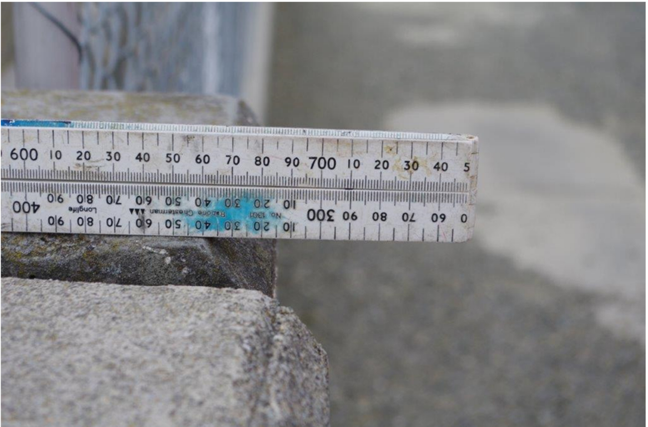
Figure 18 Offset at TL perimetric joint c2015
