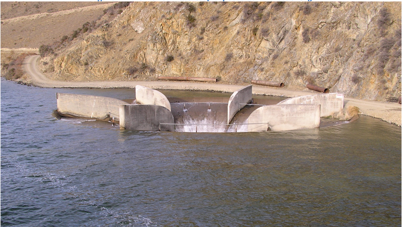
Figure 23 Partially obstructed bell mouth at track.
