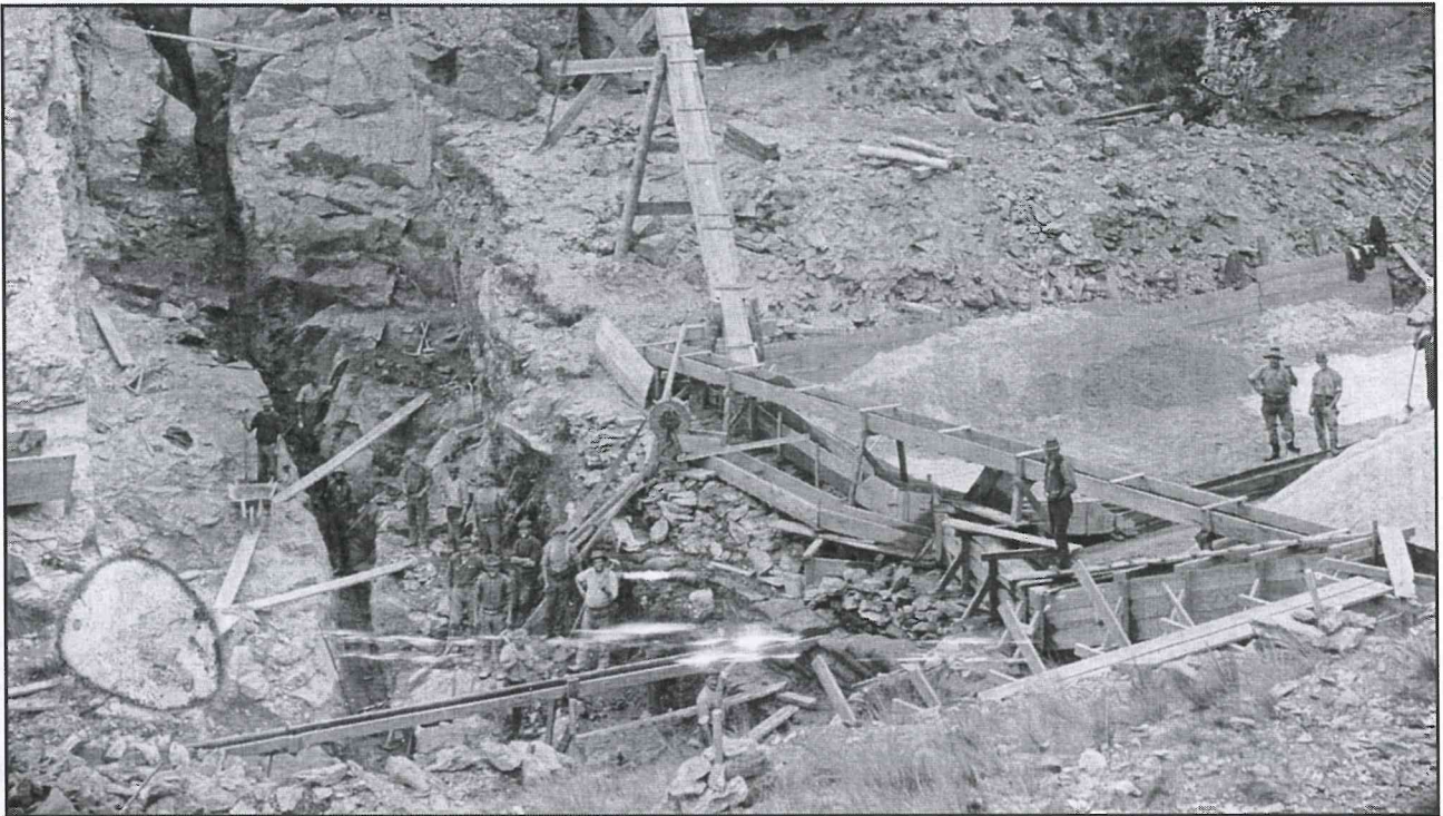
A close up of work on the fault in the base of the dam. The excavation is being done by hand tools and it would have been laborious work lifting the material out of the deep slot in the rock. On the right of the photograph is the sand cleaning operation with the shute and raw sand behind, and washed sand at the front.
