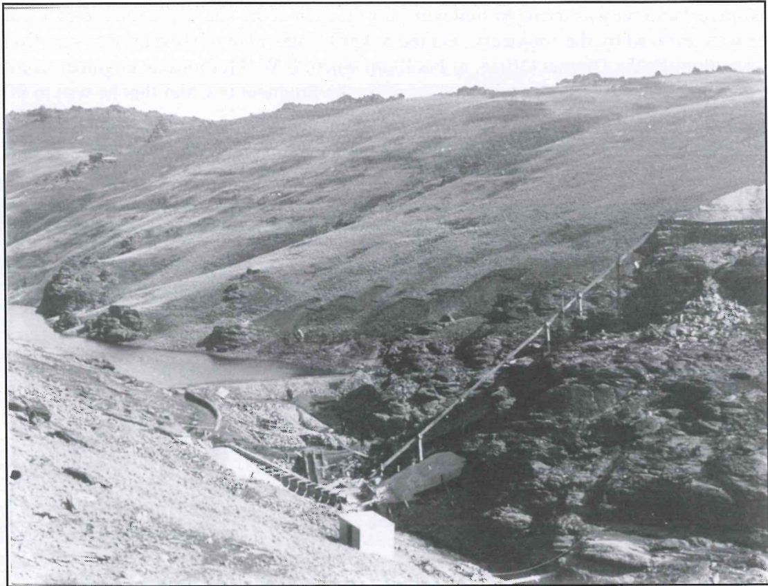
An early view of the dam construction. The upstream coffer dam is diverting the water around the right side of the valley in a race and flume. The long chute on the left bank is to allow the sand, which was being carted to the site, to be washed where there was access to water below the dam site. The dam site was still being investigated.
