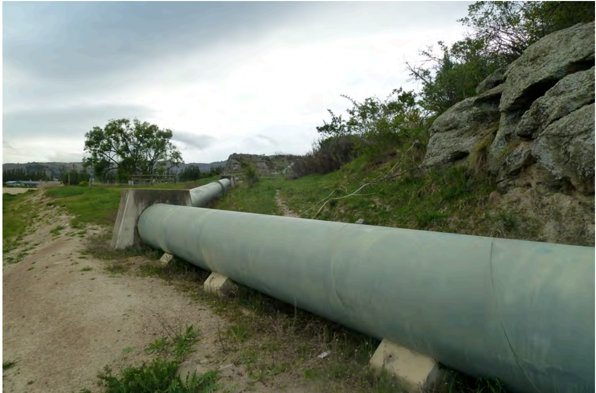
Figure 3.11: Example of pipeline similar to proposed rising main (at Strode Road Earnsclough Irrigation Co. Ltd, 28 Oct 2012)
