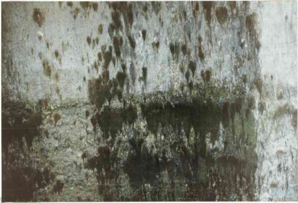
56. J# 39/40 D/S, MORE SIGNIFICANT SPALLING, NO
