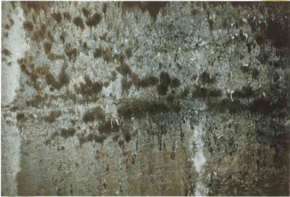
52. JF 38/39 R/S, PLASTER COULD NEED REPLACEMENT
