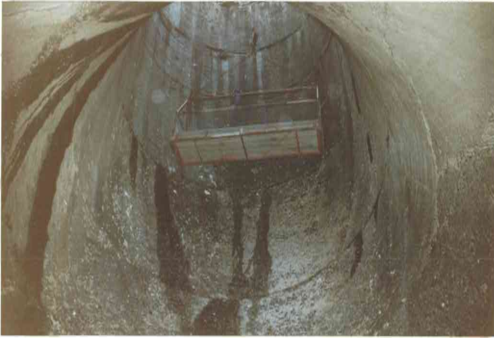
30. VIEW UP TO THROAT OF SPILLWAY SHOWING TL MID-HEIGHT CONSTRUCTION JE BUTTING UP TO JE 33/34 AT EXTREME RIGHT OF PHOTO
