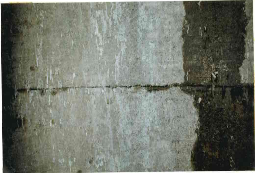
57. J# 39/40 T/L, GOOD, MINOR EROSION BELOW JE 1.5m LONG, PATCH WITH MINOR UNDERCUT.
