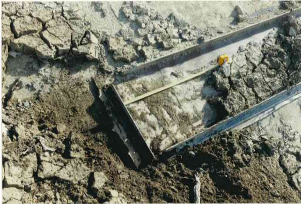
95. END OF SECOND HORIZONTAL JOINT WHERE IT COMES INTO THE TL ABUTMENT SHOWING HOW THE RUBBER STRIPS ARE HELD DOWN
