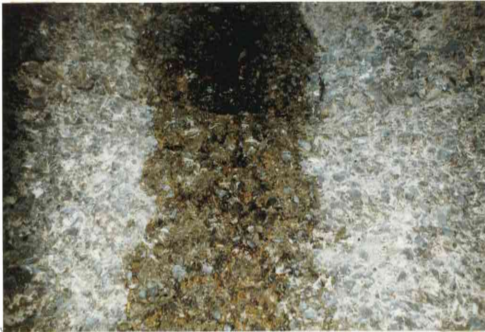
32. jt 33/34 AT INVERT SEVERELY ERODED
