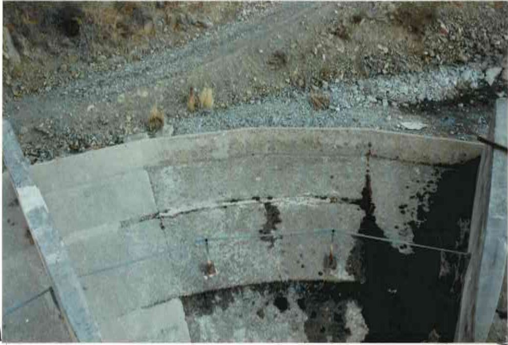
82. BAY 3, REPAIR POOR CONSTRUCTION OF MID PANEL
