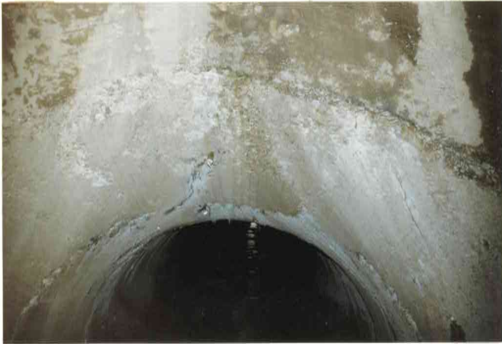
31. CROWN OF PANEL 33, OLD 19mm WEEP HOLE PIPE
