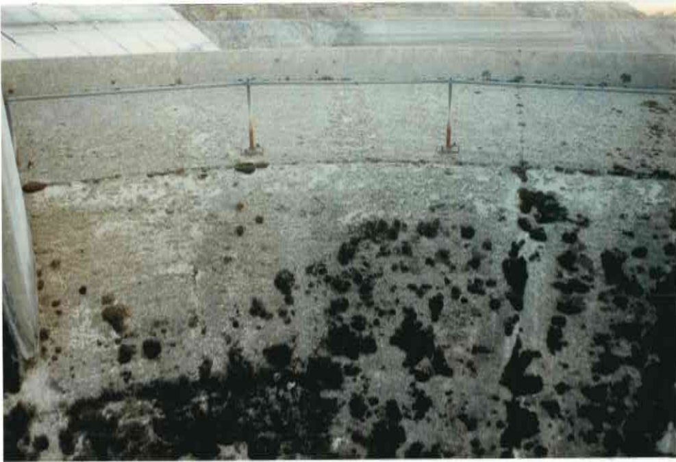
78. BAY 5, MINOR SPALLING VERTICAL CONSTRUCTION Jt. GENERALLY GOOD
