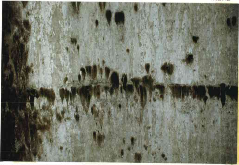
58. J+ 39/40 TR, MINOR SPALLING, SURFACE PATCHING
