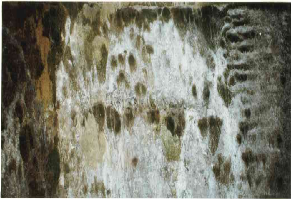
59. PANEL 40 TR DEFECT
