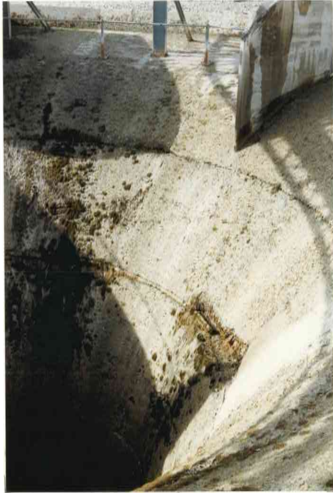
68. VIEW FROM ABOVE SHOWING DAMAGE AT JT 4/42 L/S AND TL AND AT JT 42/43 L/S
