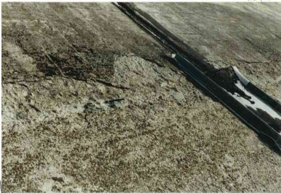
91. CLOSE UP OF SURFACE DAMAGE AT NORMAL WATER LEVEL BETWEEN FIRST + SECOND PANELS
