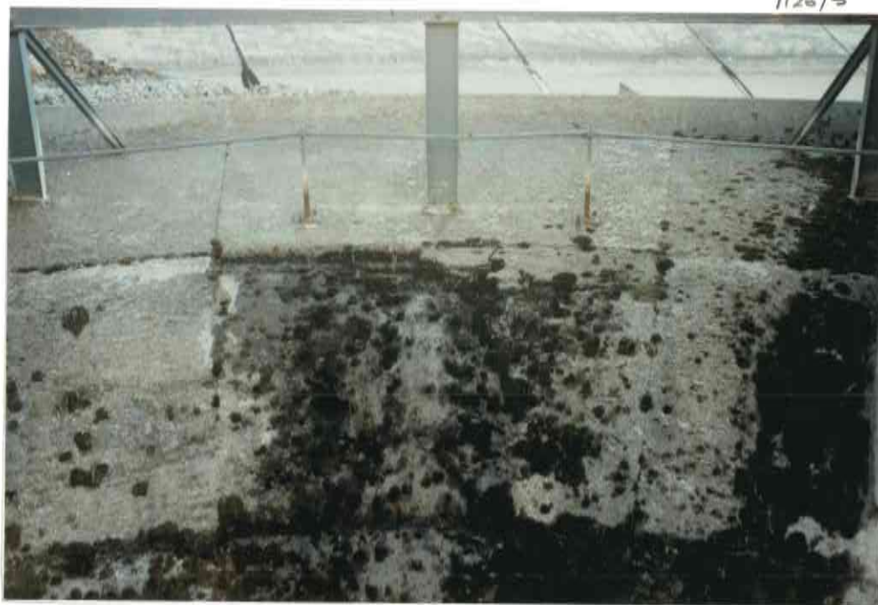
76. BAY 4 SUBSTANTIAL DETERIORATION OF CENTRAL SECTION . URGENT REPAIR
