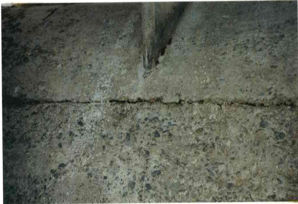
69. JT 42/43 TL, ERODED 50mm WIDE, 100-150mm DEEP
