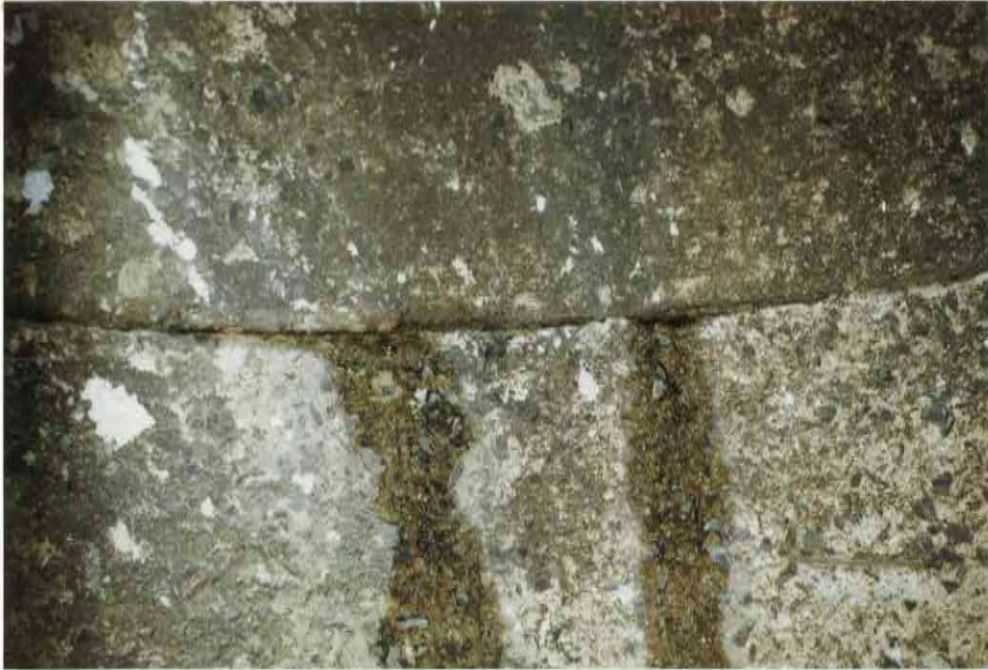
38. Jt 35/36 INVERT (U/E)
