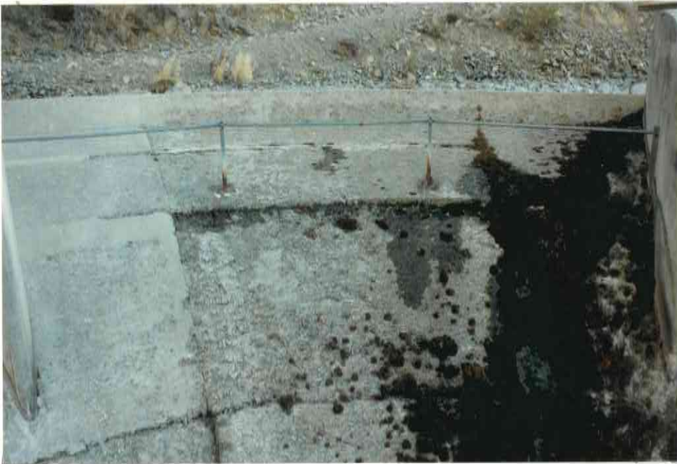
75. BAY 3 MORE SEVERE EROSION, ESPECIALLY DOWN FROM J# 43/44. URGENT REPAIR OF IT.
