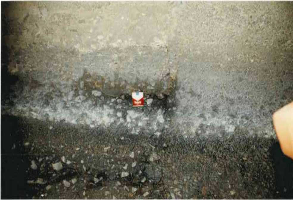
11. I/W jt TR NEXT TO JT 9/10. EROSION 150mm DEEP, 300m LONG
