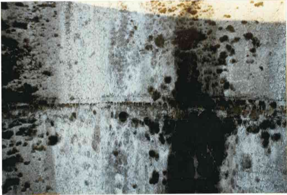
64. JT 41/42 U/S, INFILL PLASTER LOST
