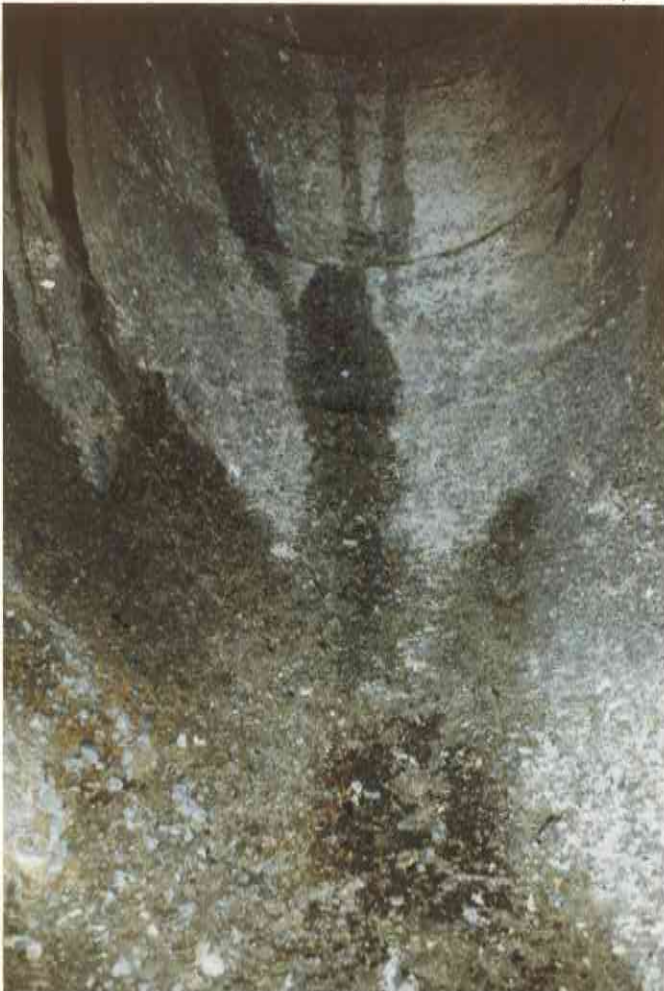
25. INVERT OF PANEL 32 IN IMMEDIATE FOREGROUND (JT 32/33 DIFFICULT TO SEE, TOPMOST JOINT VISIBLE IS JT 35/36)
