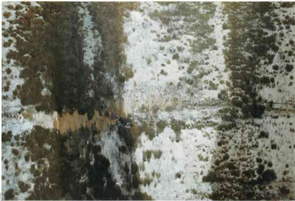
65. JT 41/42 D/S, HORIZONTAL STEEL EXPOSED, 600mm WIDE, 4m LONG + FULL PANEL DEPTH. URGENT REPAIR
