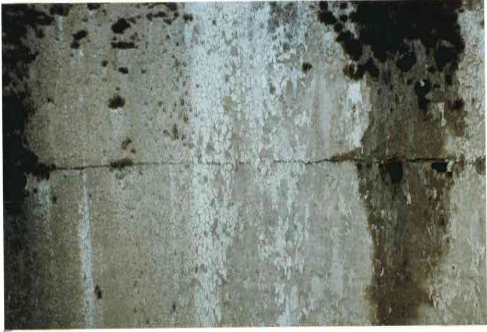
60. JF 40/41 U/S, GOOD, MINOR LOCAL SPALLING 300mm LONG
