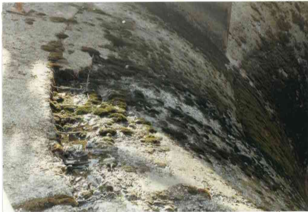
77. CLOSE UP OF DAMAGE AT Jt 43/44 BAY 4
