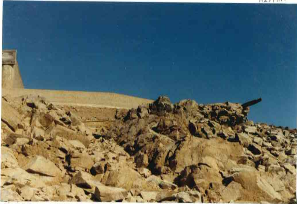
86. VIEW UP TO FOUNDATION AT BAY 5, ROCK AT CENTRE OF PHOTO MOSTLY IN SITU
