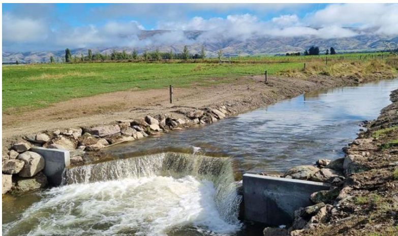
The fish barrier in Thomsons Creek near Omakau. Photo: Thomsons Catchment Project
