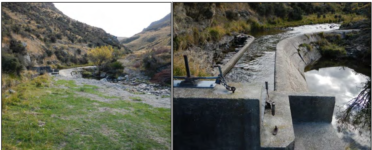
Figure 27: Omakau Irrigation Scheme – Thomsons Creek intake.
