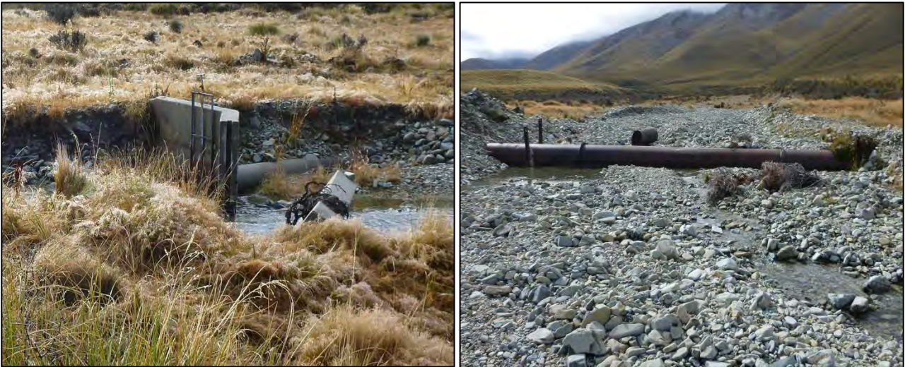
Figure 35: Mount Ida Race: Johnstons Creek (top end) intake weir and Kirkwood Creek Siphon.
