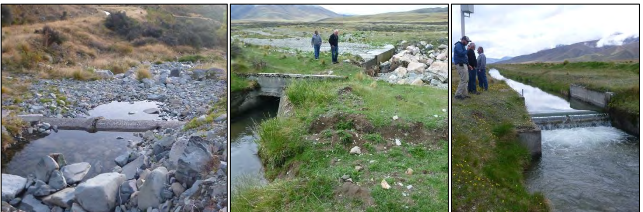
Figure 37: Mount Ida Race: Healeys Creek Siphon, Hills Creek Siphon and Johnstones flow monitoring weir.
