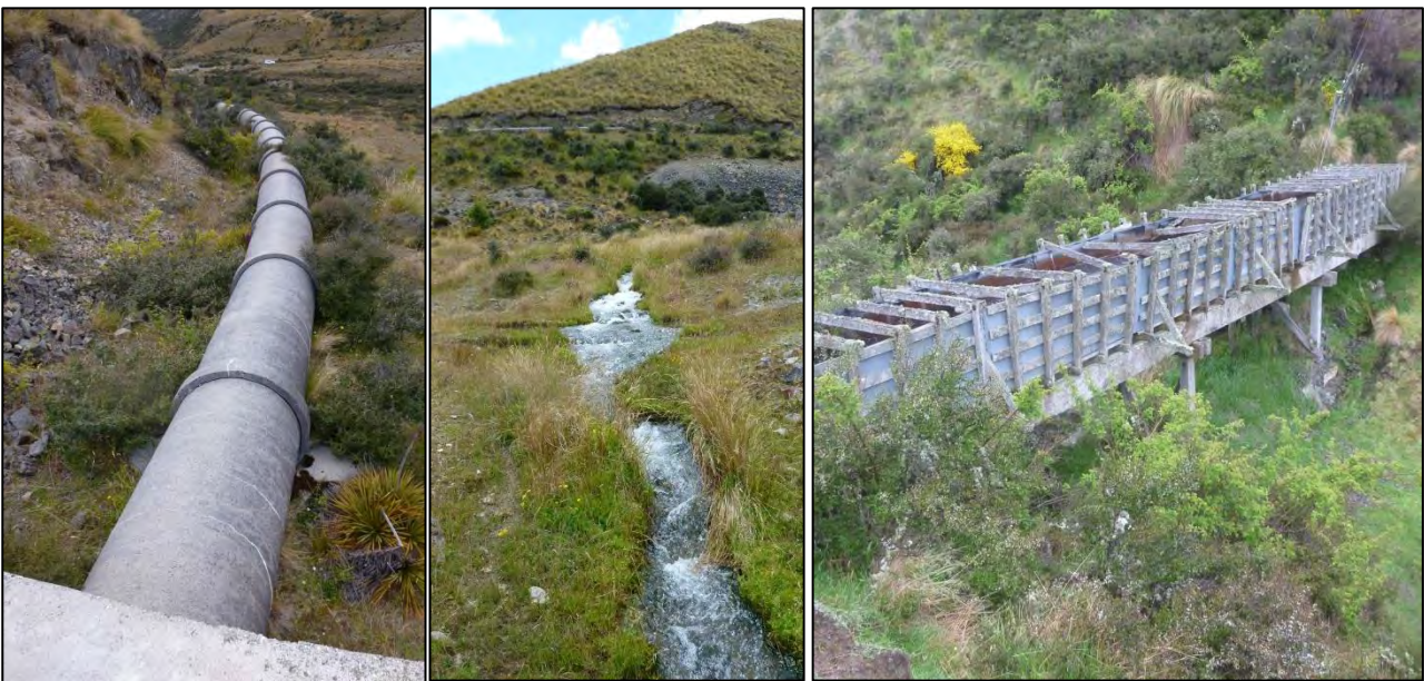
Figure 36: Mount Ida Race: Hut Creek Pipe, pipe leakage and Scotts Flume.
