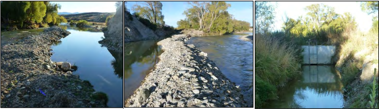
Figure 21: Blackstone Hill Irrigation Scheme River Intake.
