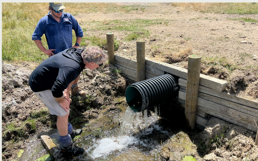
Perched culvert to protect upstream galaxias population in this small tributary
