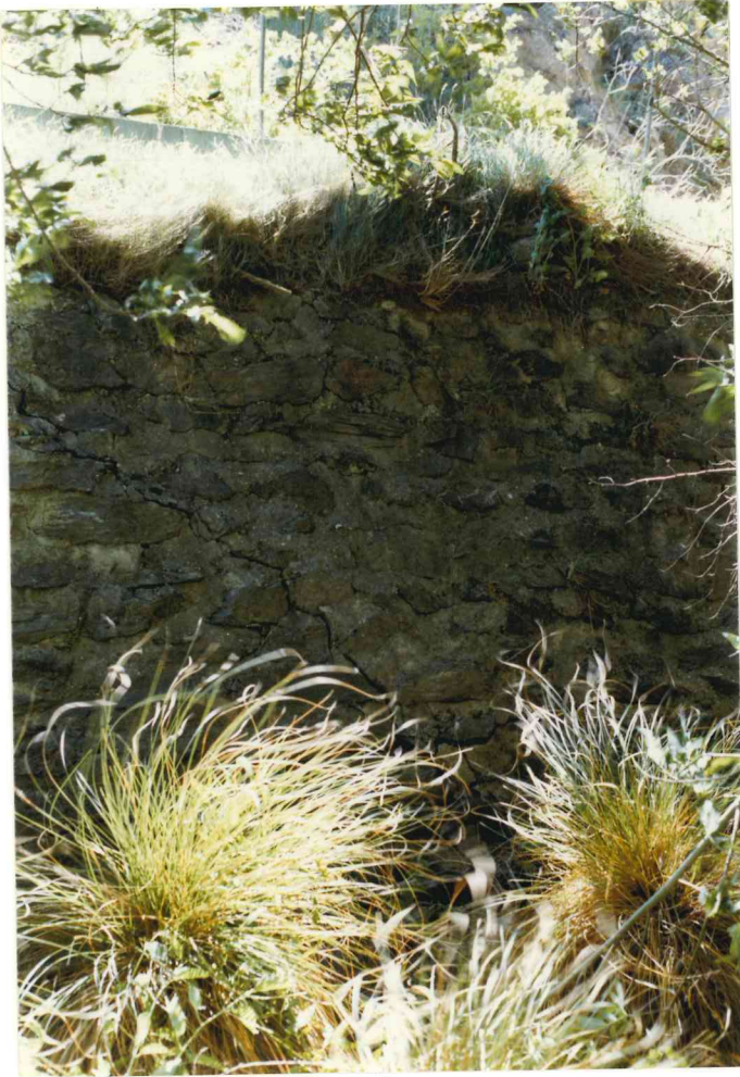
Plate 6 Cracks in Handplaced Rockfill (Indicates Deep Seated Movement)
