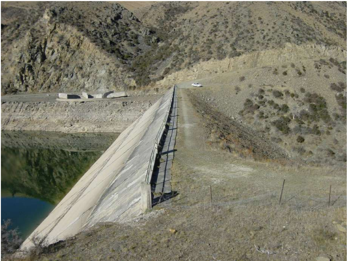
Figure 24 Dam Crest Deformation
