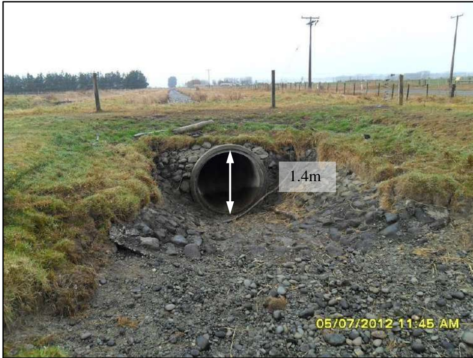
Figure 23: Example of a pipe culvert farm track over a 1.8 \text{ m}^3/\text{s} race
