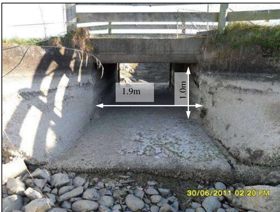
Figure 22: Example of a box culvert farm track over a 6 \text{ m}^3/\text{s} race
