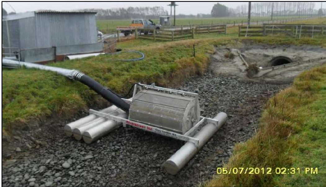
Figure 26: Example of pumping from a race with a screen on a pontoon.
