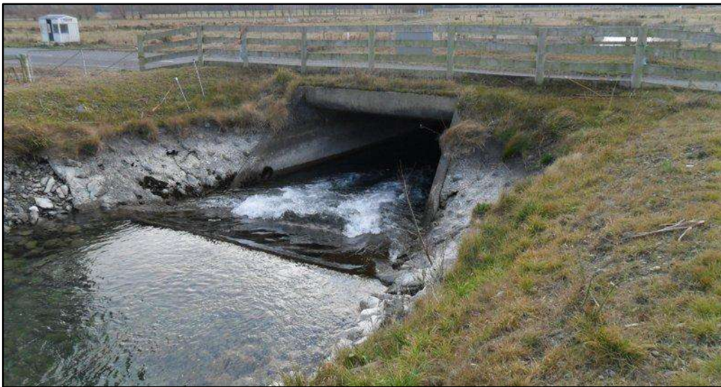
Figure 21: Example of a box culvert road crossing over a 13 \text{ m}^3/\text{s} race
