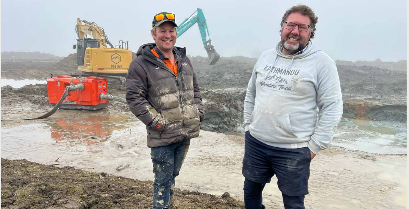
S&B Civil's Cody West and Thomsons chairperson Hamish Stratford on site during construction.
