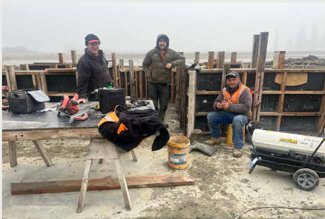
Ross Mitchell, Kirk Samuel and Dick Brown from Breens constructing the exit weir.
